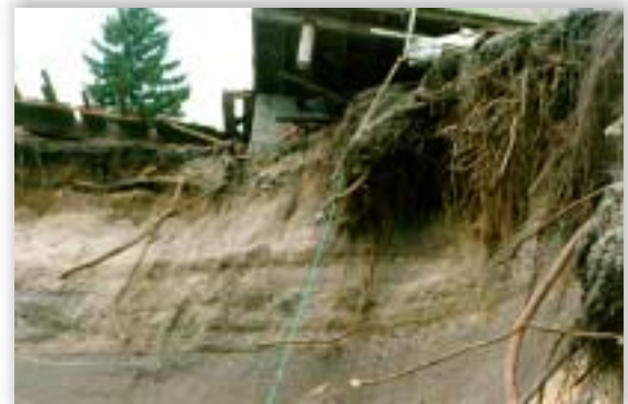
Figure 30 - Wind Erosion Damages on Soft Sand
